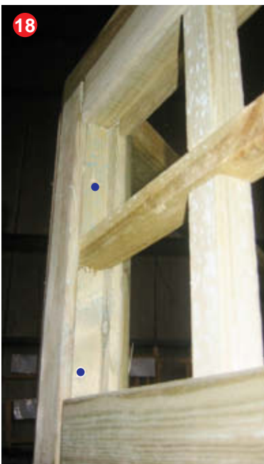
18 Secure fence with 4 x 50mm screws, 2 at each end of the fence.
