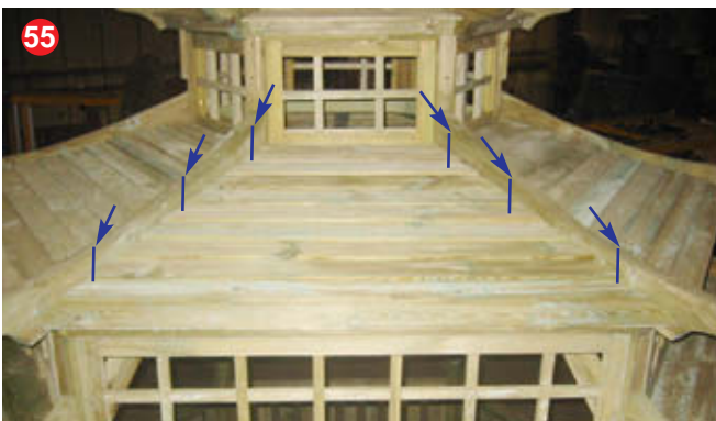
55 Secure the panels on the middle roof bearers using 6 x 50mm screws.
